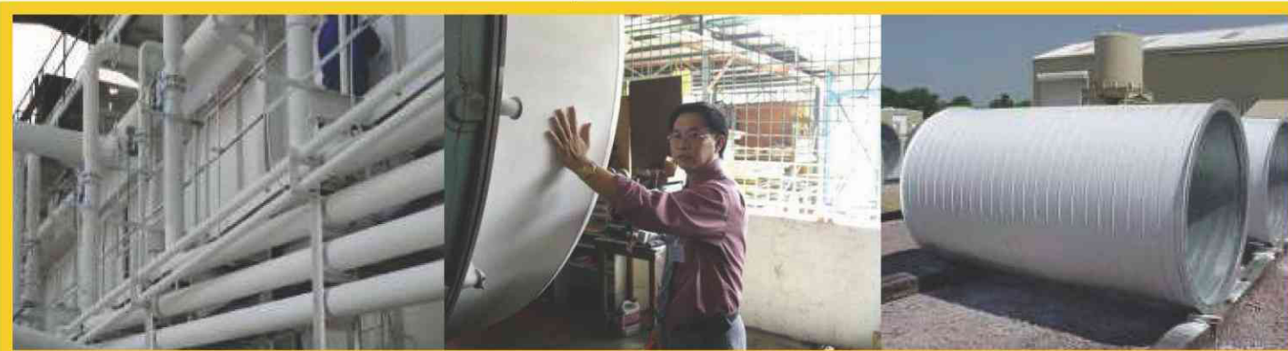
Thermal Insulation Various piping
